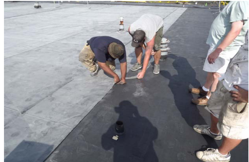
Another view of the backing paper being pulled from the seam tape.
