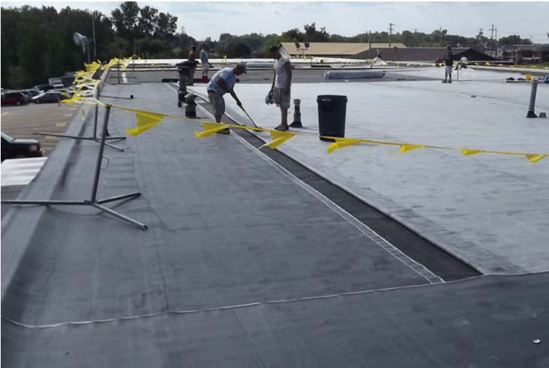
Another view of the top membrane folded over and being cleaned while the seam tape has already been put down.
