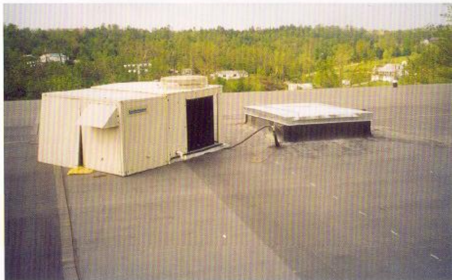
Tornado winds blew the HVAC unit off the curb as the 2001 Company system sucked down tight.
